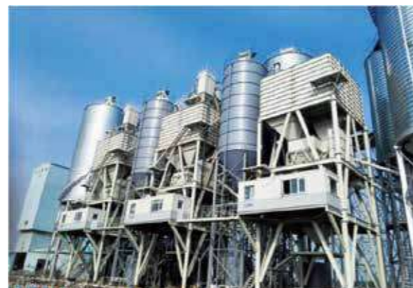
广州长丰3HLS270V(环保搅拌楼) 3HLS270V (environmental mixing tower) in Guangzhou
